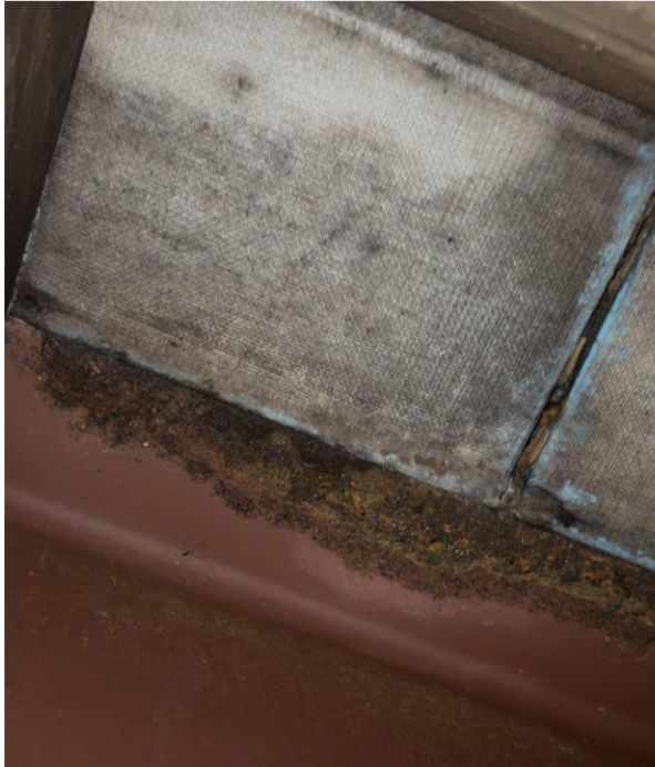
Photo 13 — Beam top surface with mineral residue and corrosion
