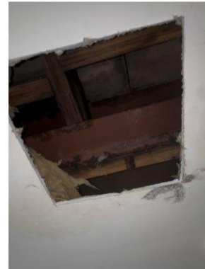
Photo 8 — Second inspection opening — extent of cavity damage
