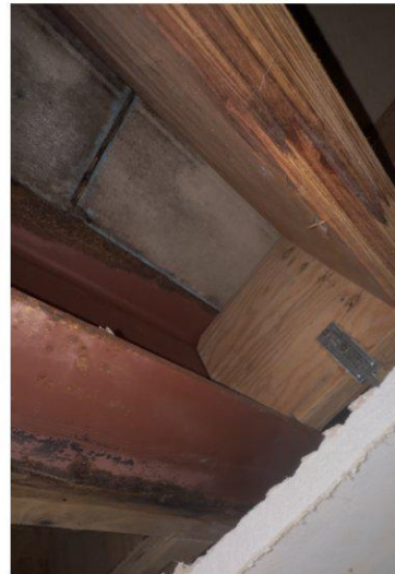
Photo 12 — Cavity view showing contaminated insulation and damp framing
